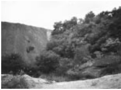
Unvegetated slag slope meets a vegetated slag slope. Same exposure, same angle of repose, different grain size. More construction debris on the right slope.
